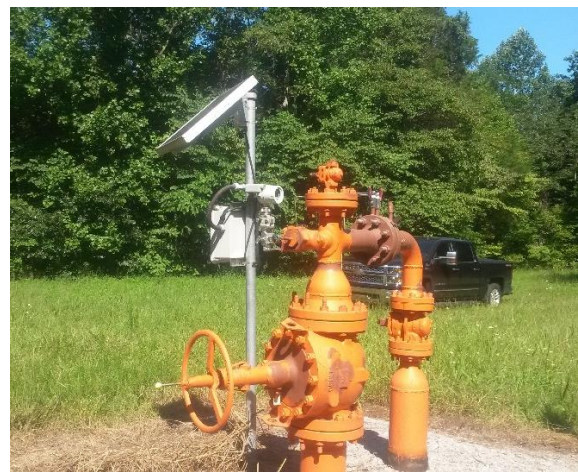
Figure 6: Wellhead transmitter powered by Solar Panel
