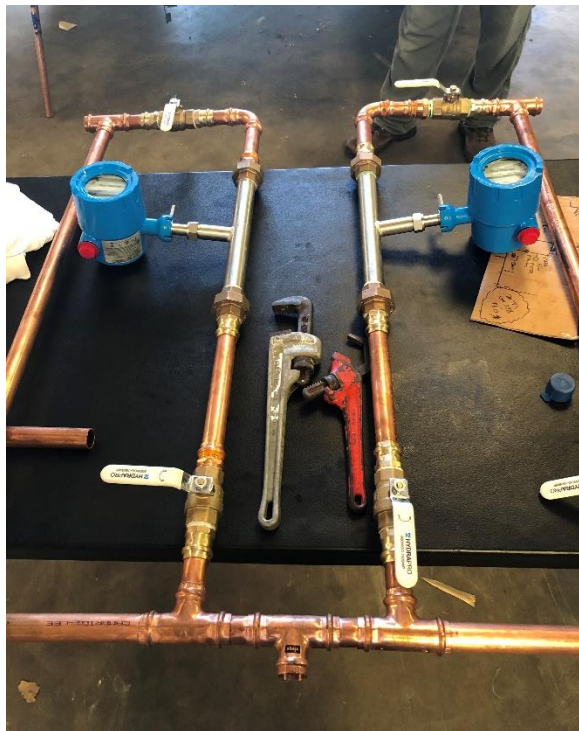
Figure 5: On-site startup support quickly corrected a flowmeter installed in the wrong direction.
